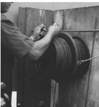
5. For additional stability, it's necessary to secure the sleeve with wire to the rebar. Insert the other end cap firmly, check that second end cap is positioned correctly, confirm sleeve length and close the form.
